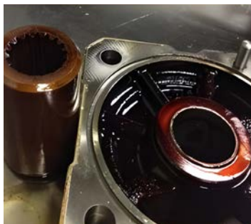
Varnish on housing cover of hydraulic pump
