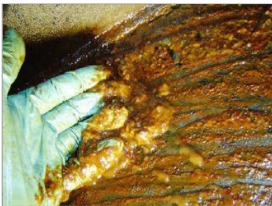
Photo 1 Effect of Electrostatic discharge within hydraulic fluid system, resulting from rapid oil aging rate in formation of sludge.
